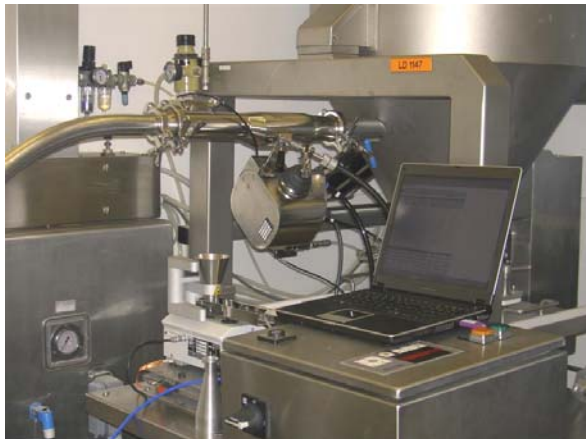
Figure 7: Very narrow conditions for a \varnothing 50 mm sampler TWISTER and GMP-Module; analyser within a mobile rack
